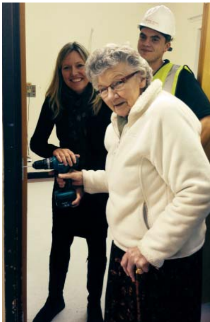
Ruth Wright (front), one of the longest-serving members of the League of Friends, starts the work on the £135,000 building project at Ottery St Mary. Also pictured are Gaynor Appleby, manager of the Rowan and Linden centres, and Karl Thomas from building contractor Hodges, Bridle and Co Ltd.
