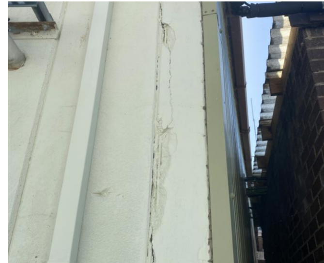
Form of Construction Photo 3 Photo at location of spalling showing reinforcement. No signs of corrosion to exposed reinforcement.
